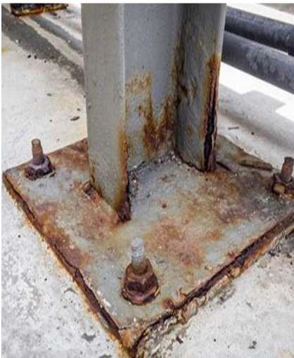
Rust at the base of the canopy
