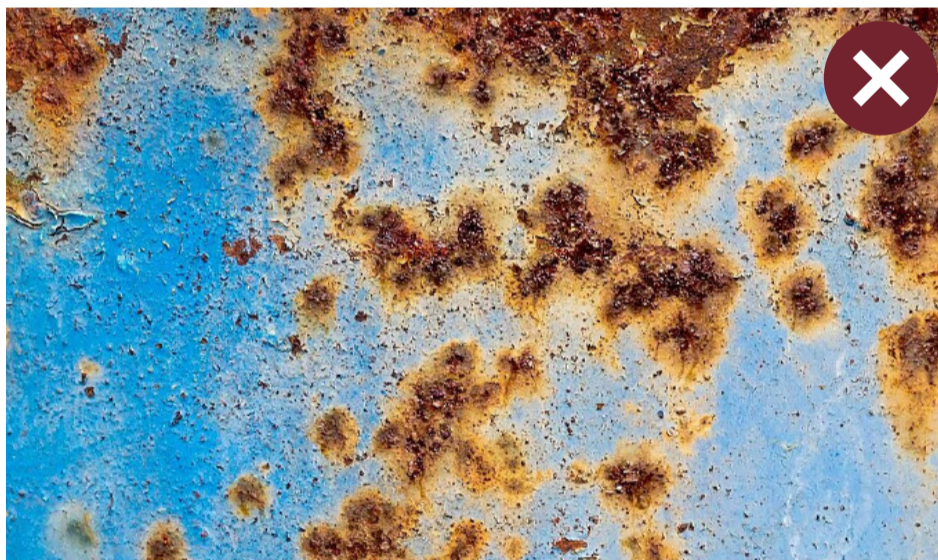
Figure 2.38: Peeling & Rust of the Painted Metal Finish
