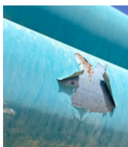
Peeling in the paint
