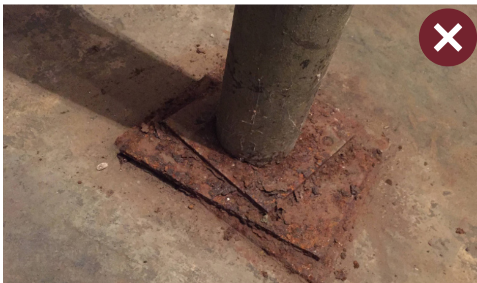
Figure 2.39: Rust at the Base of the Shade Structure Column
