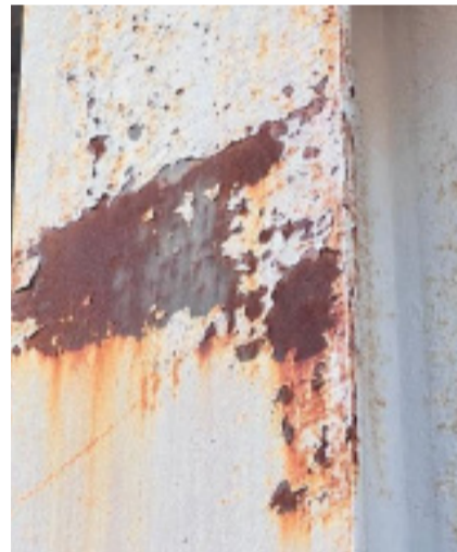
Rust in canopy columns
