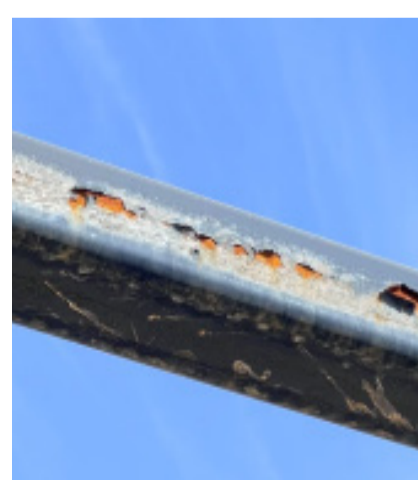
Rust in canopy bridges
