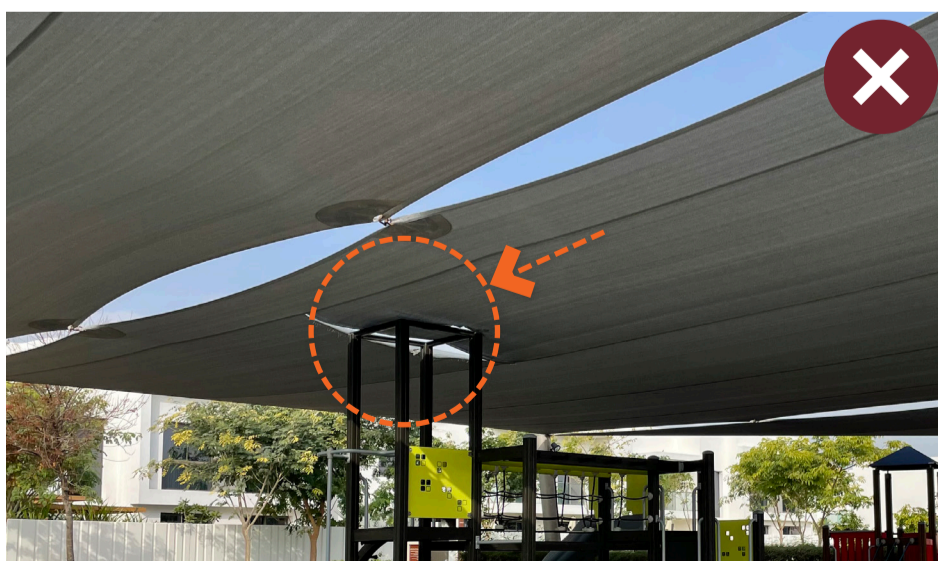
Figure 2.30: Shade Structure too low for purpose
