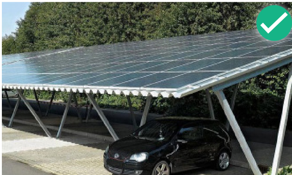
Figure 2.31: PV-Panel Car Parking Shade Structure
