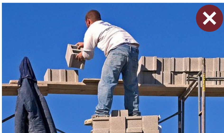
Figure 2.36: Unsafe construction conditions
