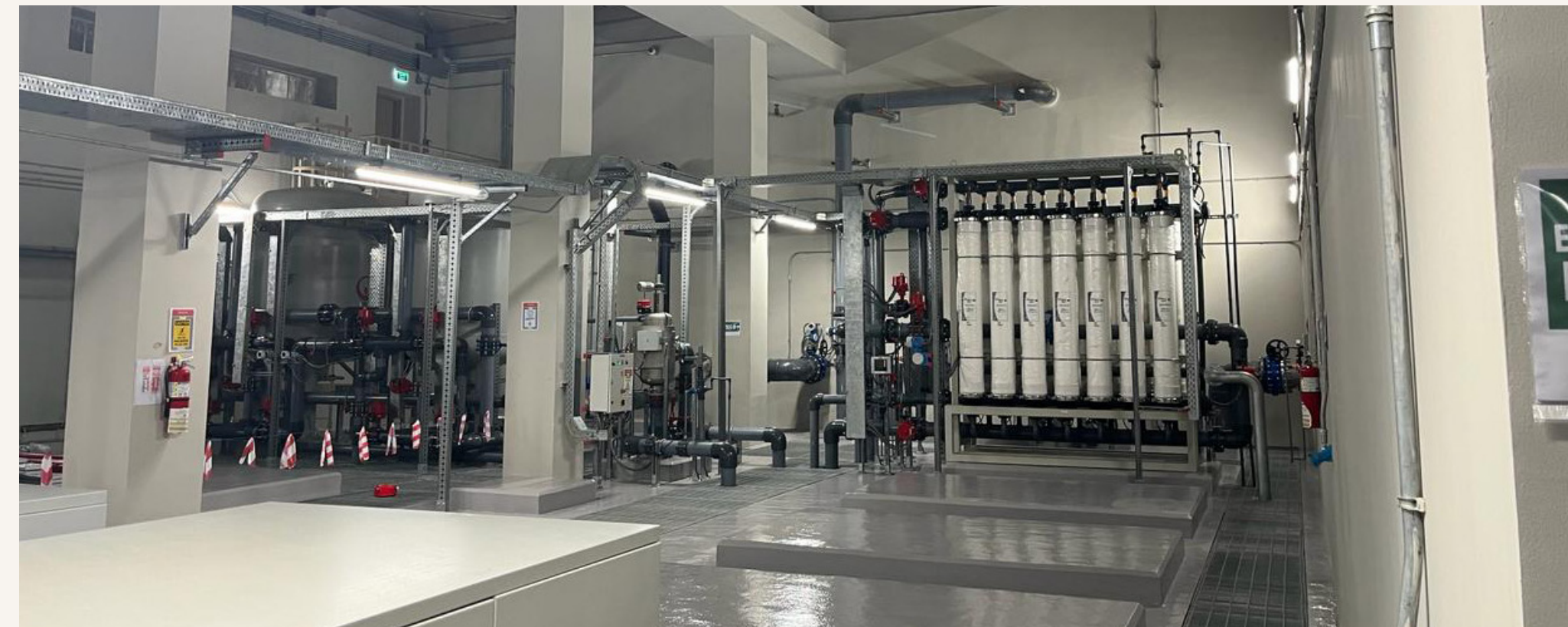
Water Treatment Plant - Ashar Valley
