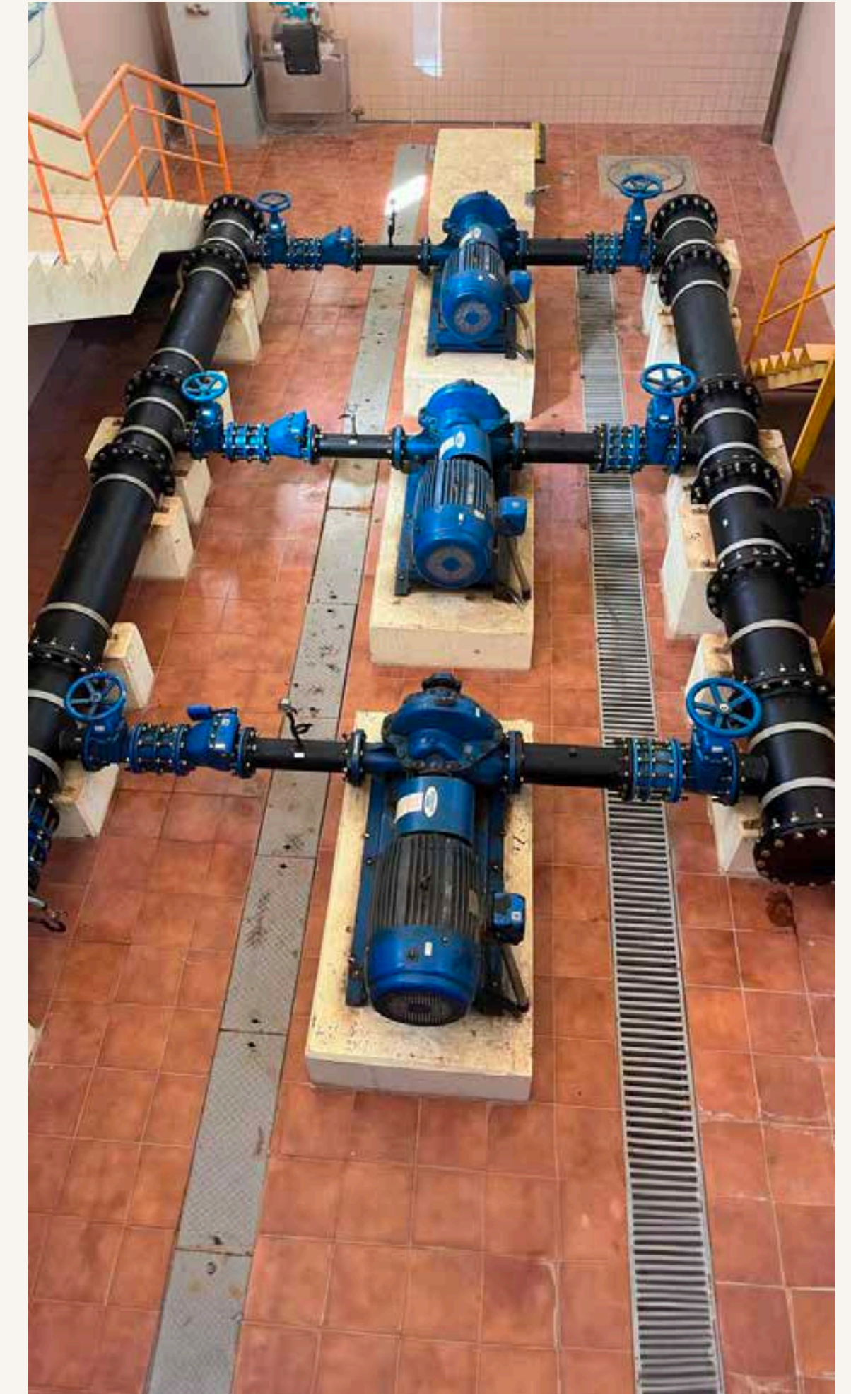
Water treatment facility - Ashar Valley
