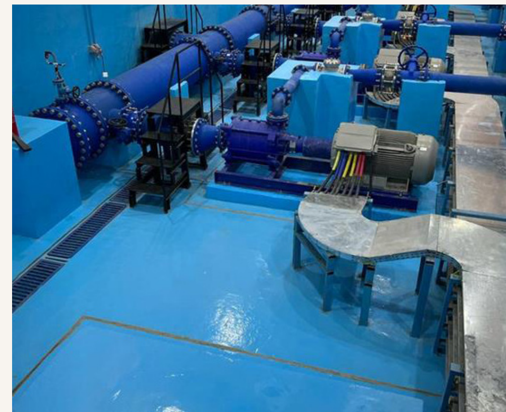
Water treatment facility - Sharaan
